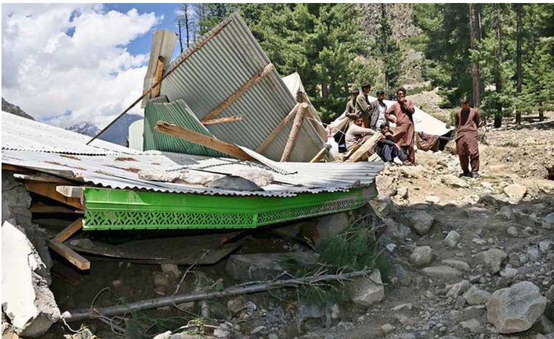
Houses and infrastructure in the ‘Dalan’ area of Naltar Valley have collapsed or sustained severe damage due to recent flash floods, while affected residents await government assistance.
