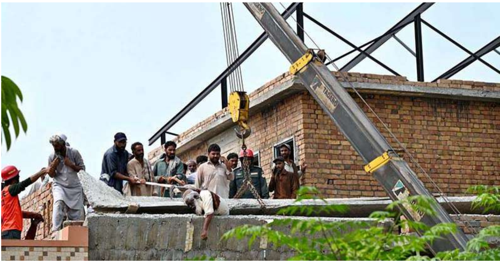
A daily-wage labourer was killed when a concrete shade collapsed on him at an under-construction house in Media Town. Rescue teams retrieve the body from the debris.
